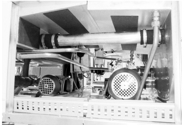
Overflow pipe between the final rinse tank (on the left) and chemical wash tank
